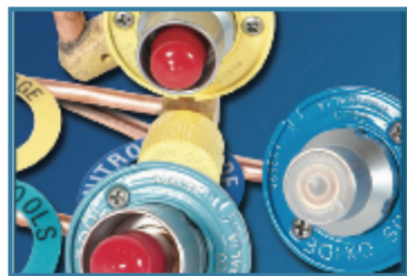
Medical Gas Outlets fitted on Plastic Accessory Mounting Plates
